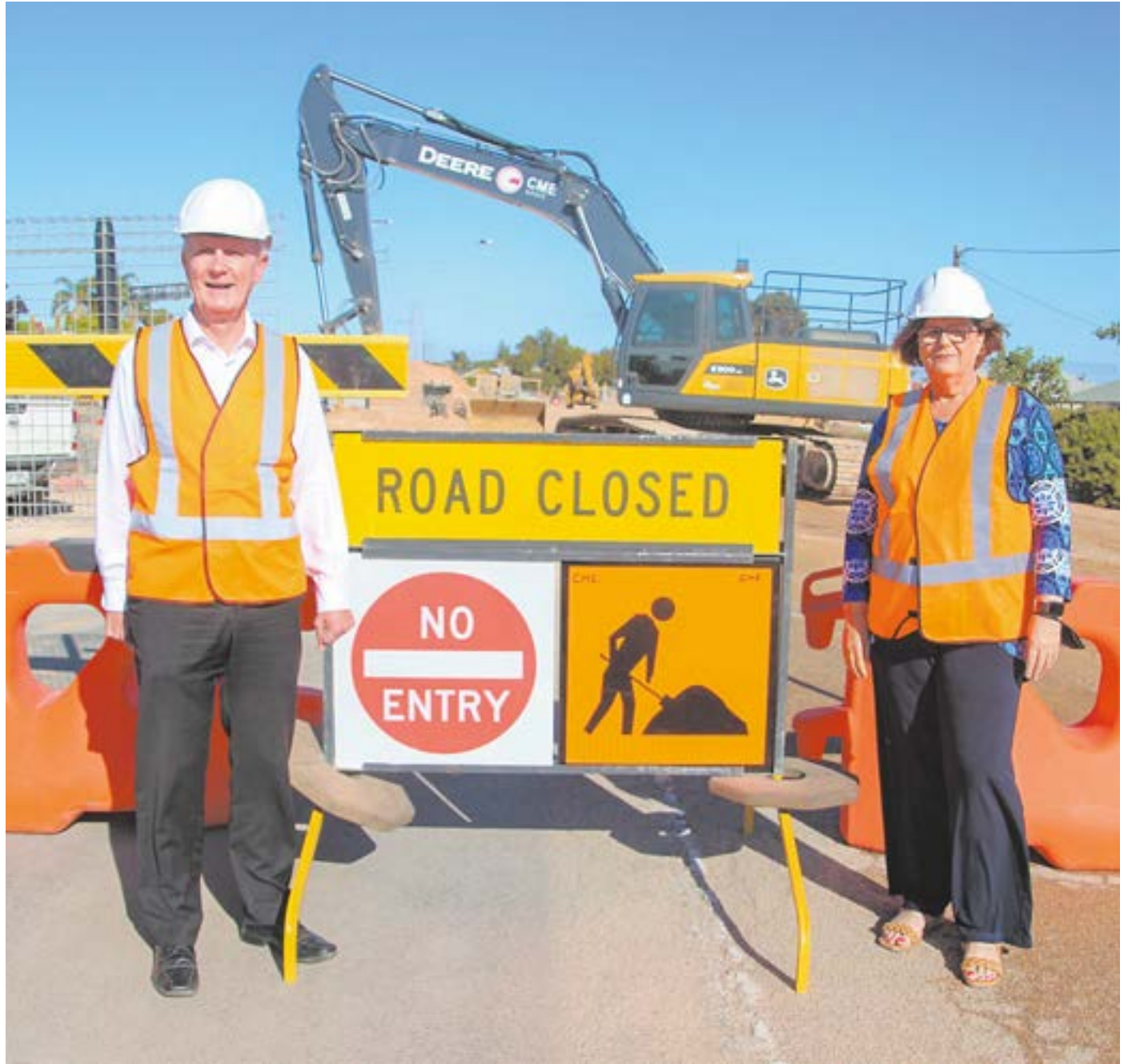
BAY ROAD... Copper Coast Council CEO Russell Peate and mayor Roslyn Talbot are pleased with the progress of the Bay Road, Moonta Bay, upgrades and said the road would be cleaned and open for the Christmas holidays before work started again in the New Year.
