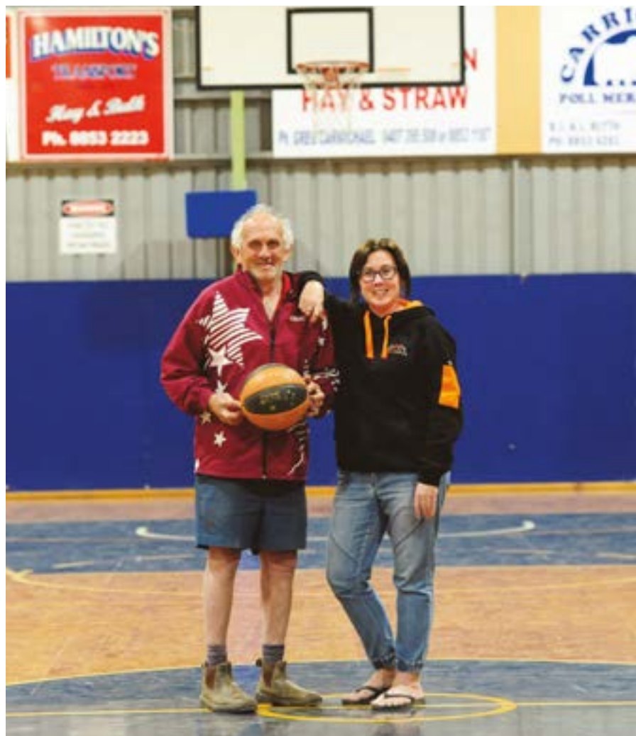
NO MORE LEAKS... Former SYP Basketball Association president Ivan McMahon with Kelly Porter underneath the newly installed roof section at the Minlaton indoor stadium.
